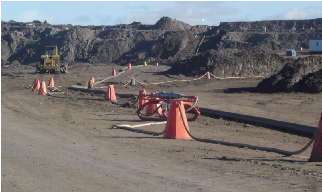
Heavy Duty Rocking Horse Skid with Strain Relief shown in service in the Alberta Oil Sands. (Also shown: UCS30/Orange, Universal Cable Stands)
