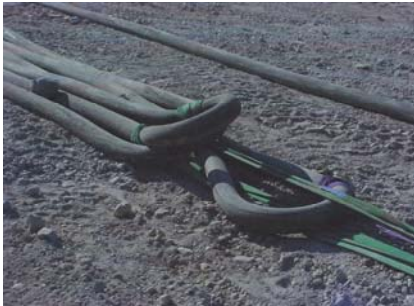
Improper method of cable dragging
